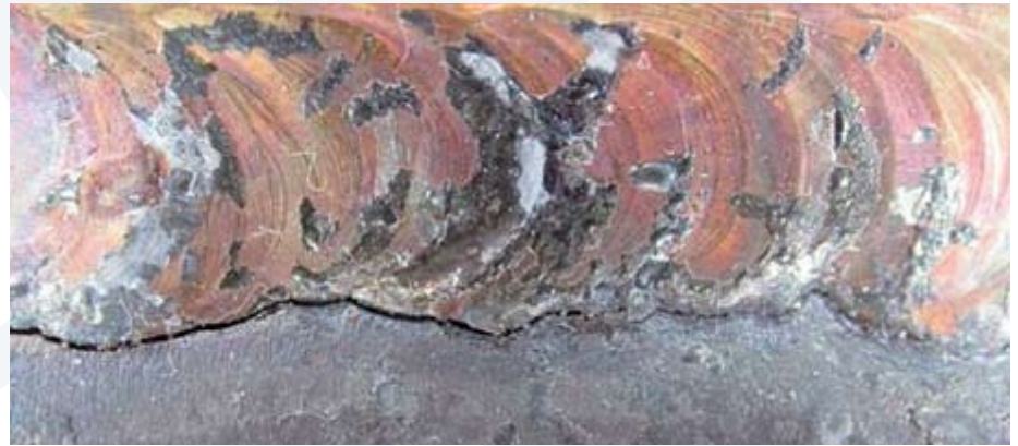
Figure 1: Welded brackets with cracks along the welding.
