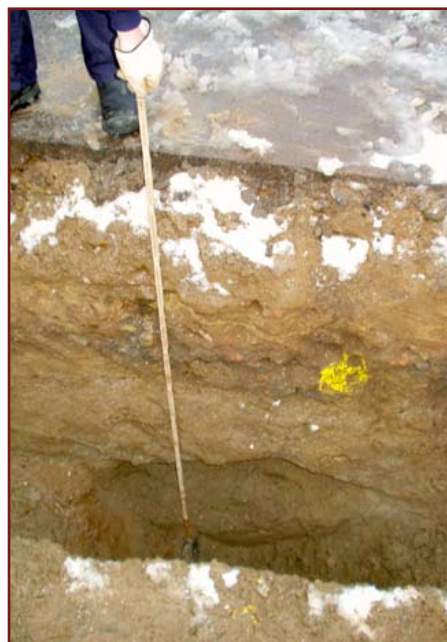
The pipe is located in a depth of 1.8 m and with an accuracy of 20 cm.
