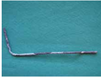
Example of wire tie of hot-dip galvanized steel after about 30 years. Very deep corrosion attacks at bend and in straight piece.
