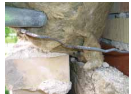
Housing association Fjordblink. Galvanized tie is almost corroded through. Photo courtesy of Grontmij A/S in Aalborg.
