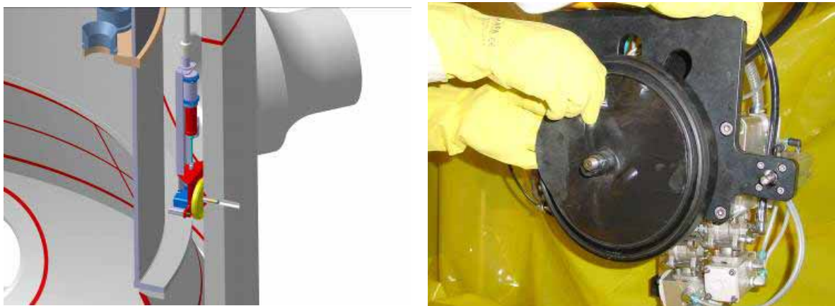
Figure 4. The remote application tool is shown fixed in the level measuring nozzle at a water depth of 26 meters. The yellow part forms the outer mould and the component form the inner mould.
