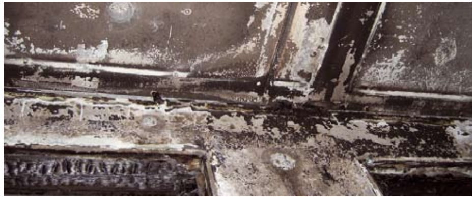
Repercussions of a massive fire impact on concrete surrounding a window opening.
