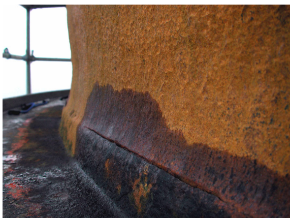
External corrosion appears after removal of the jacketed insulation
