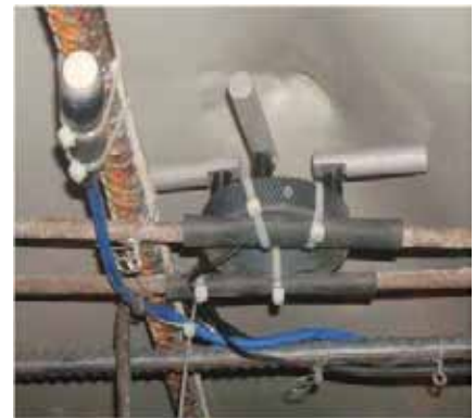
Figure 3: Typical installation of a CorroWatch sensor and an ERE 20 reference electrode.
