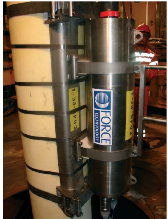
Touch down area controller with Sicon delivered modem units.
