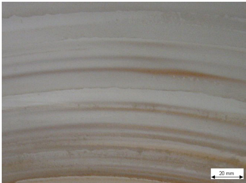
FIGURE 4 – Rouge in a WFI buffer tank. As a result of an alternating water level, rouge has deposited on the shell in circumferential areas of varying height.
