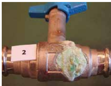
Heavily corroded valve, only a few years old
