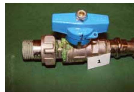
Heavily corroded brass valve
