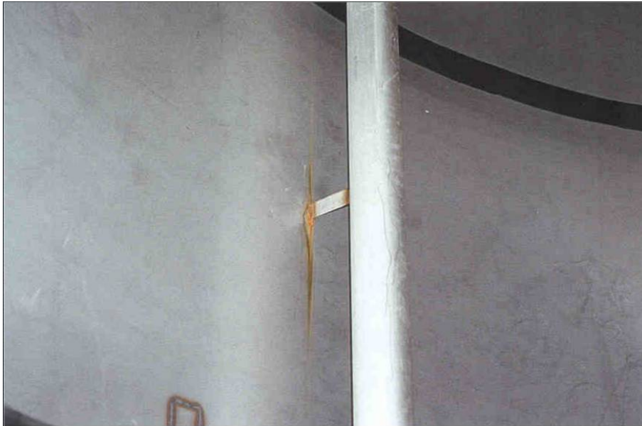
FIGURE 7 – Severe pitting in an AISI 304 cold water tank caused by lack of final surface treatment of the weld between the tank shell and the flat iron used for attachment of the inlet pipe. Moreover, pitting was also observed in a heat tinted area on the tank shell as a result of lack of post-treatment after external welding of support for a rectangular hollow section.
