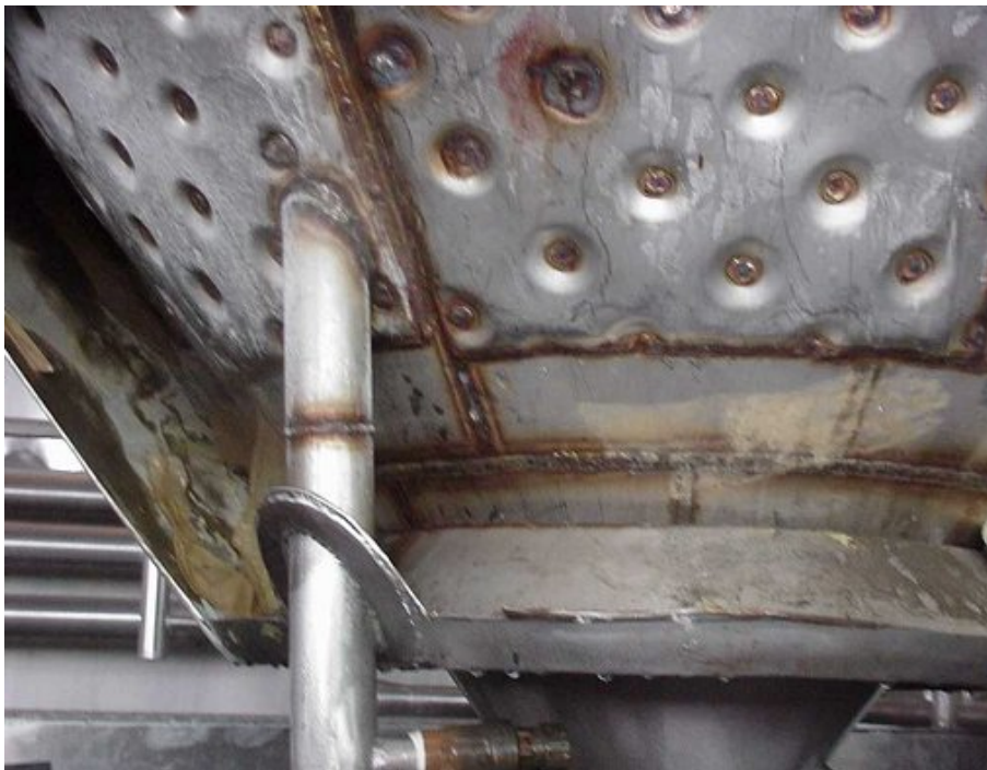
FIGURE 14 – Overview of the bottom of the yeast storage tank after removal of the insulating material. The great majority of the repair-welded dimples were observed in clusters. Unlike the original welds at the dimples between the jacket and the tank bottom, it seemed that the repair welding had been performed using filler material.
