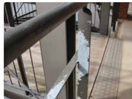
One year old Duplex system painted with alkyd-paint has been destroyed. Cost for repair, more than DKK 50,000.
