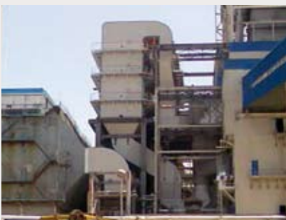
Full scale SCR unit constructed at power plant.
