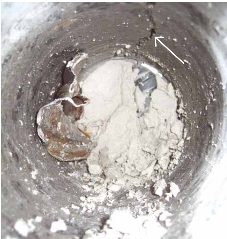
Core drilling in column showing separated material in the corrugated metal duct, i.e. cement paste. The crack is caused by frost burst in the corrugated metal duct.
