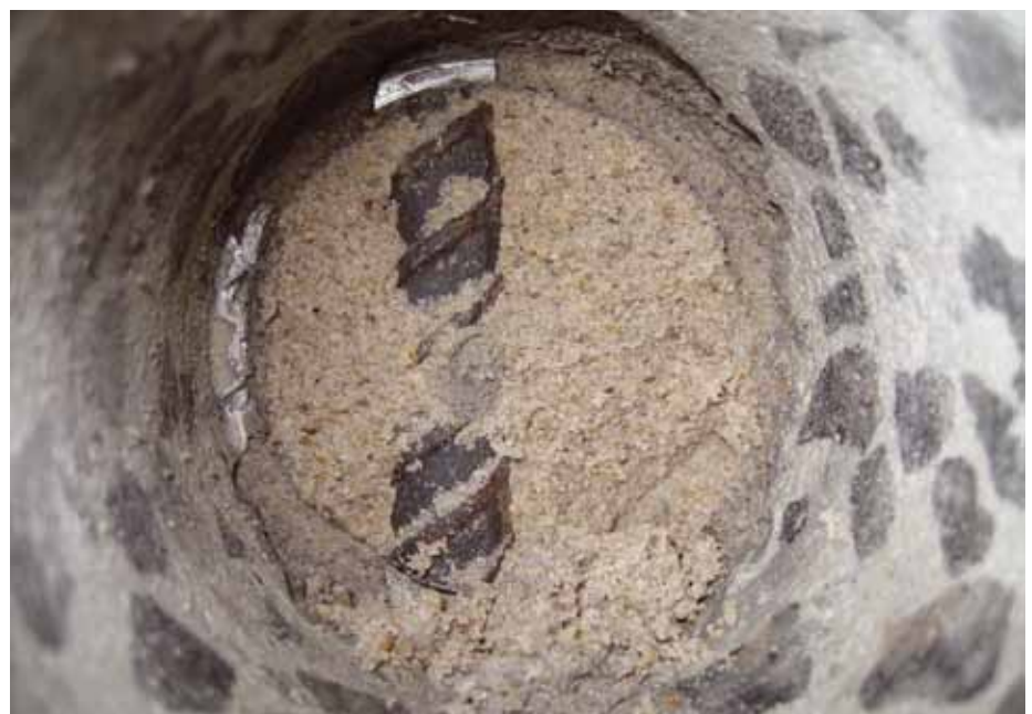
View in perimeter column showing granular material in corrugated metal duct, i.e. incoherent sand-like material.
