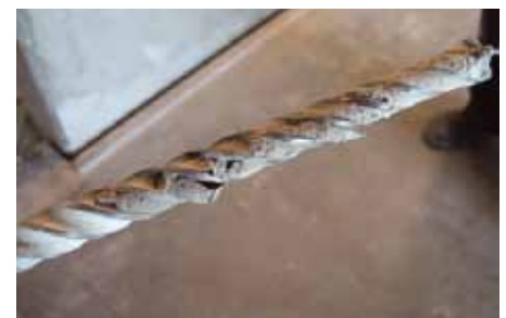
Test drilling where nondestructive measuring has localised faulty embedding. Wet/moist grouting material and not dry drill dust may be seen on the shown 12 mm drill bit.
