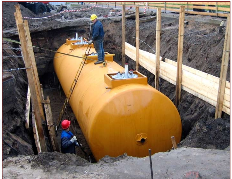
FORCE Technology assist at determining the correct surface treatment of embedded tanks to avoid corrosion.
