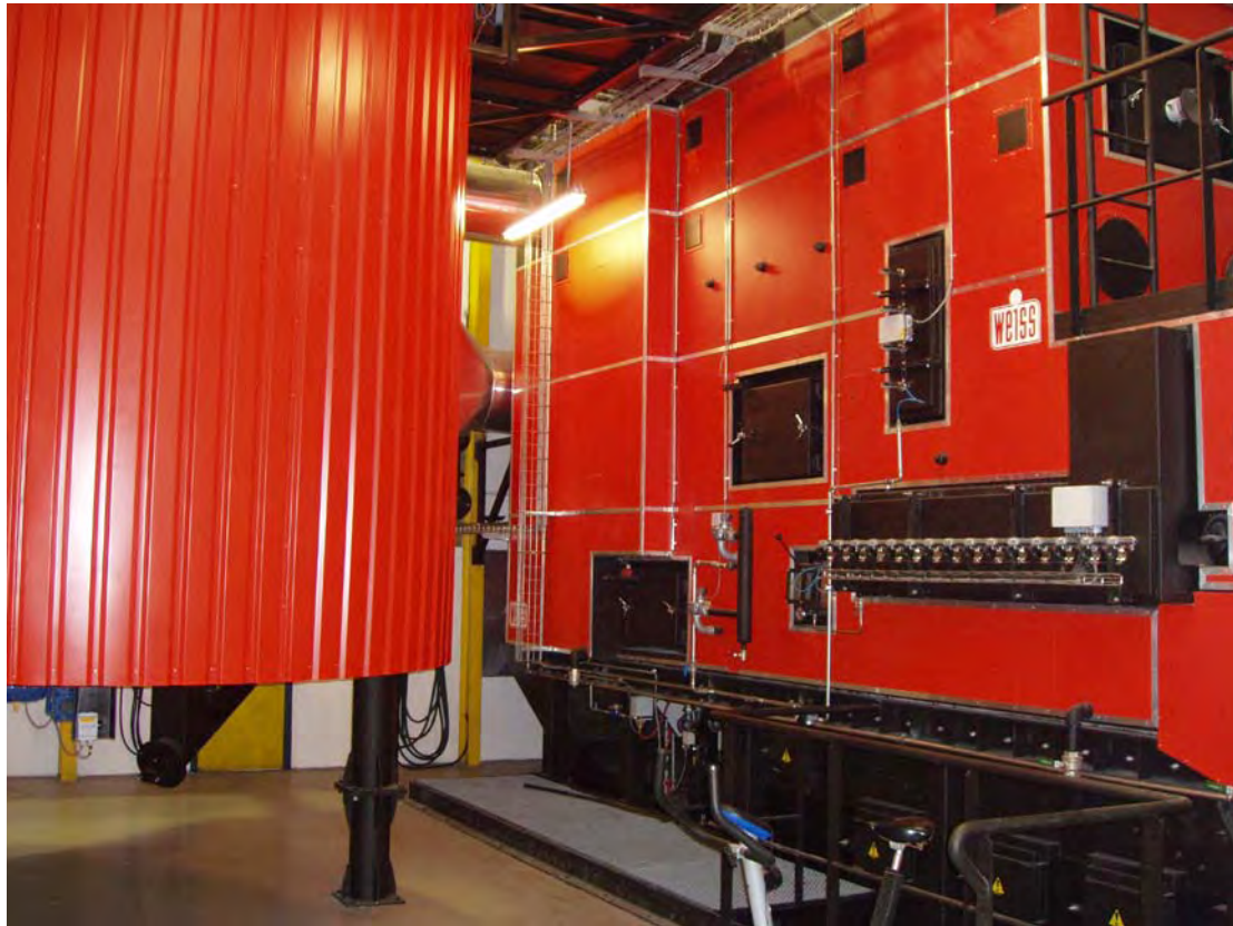
Furnace and boiler section to the right, and bag filter to the left
